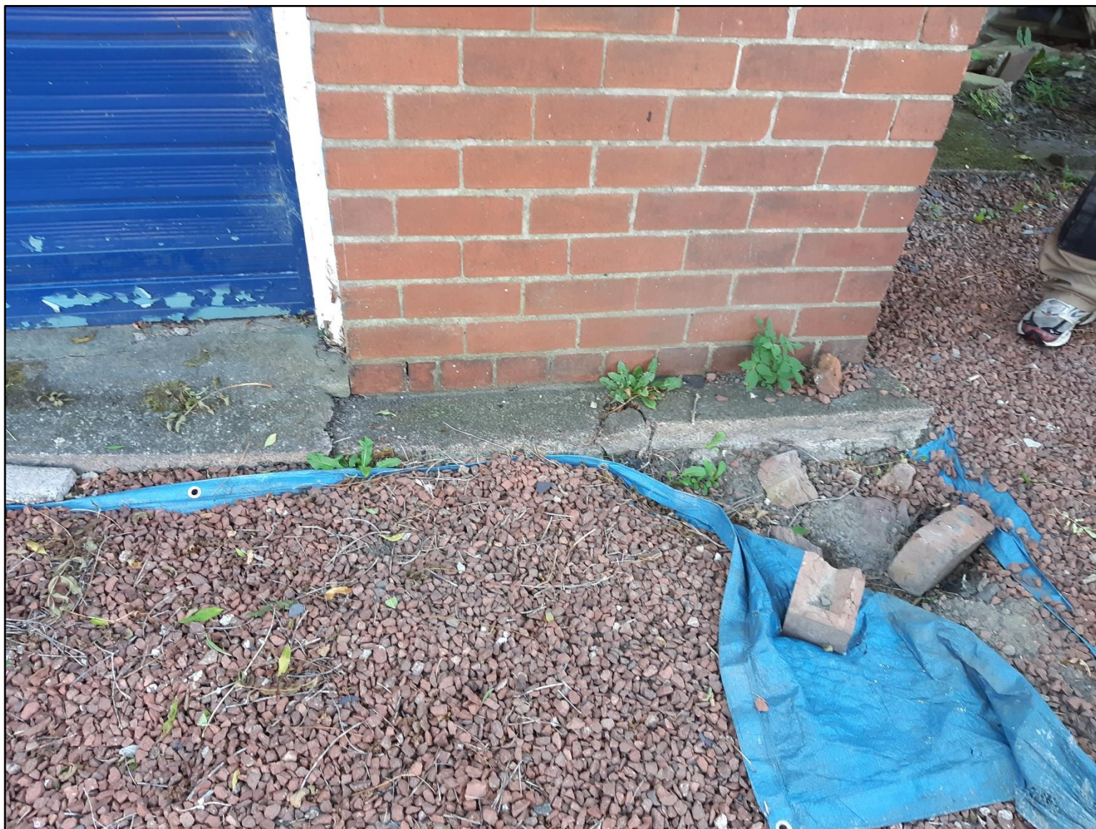
Photo 9 – Cracking & fragmentation of concrete pad
