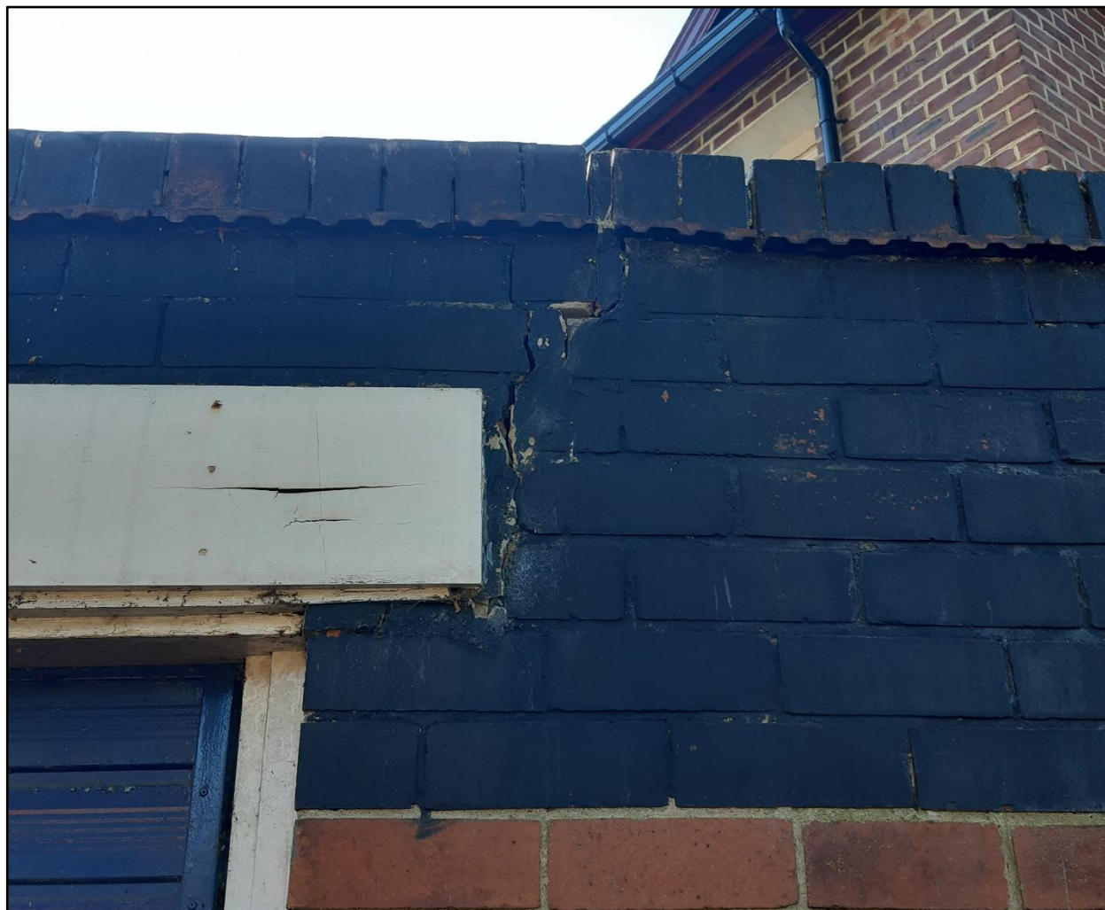
Photo 10 – Cracking adjacent to lintel on garage
