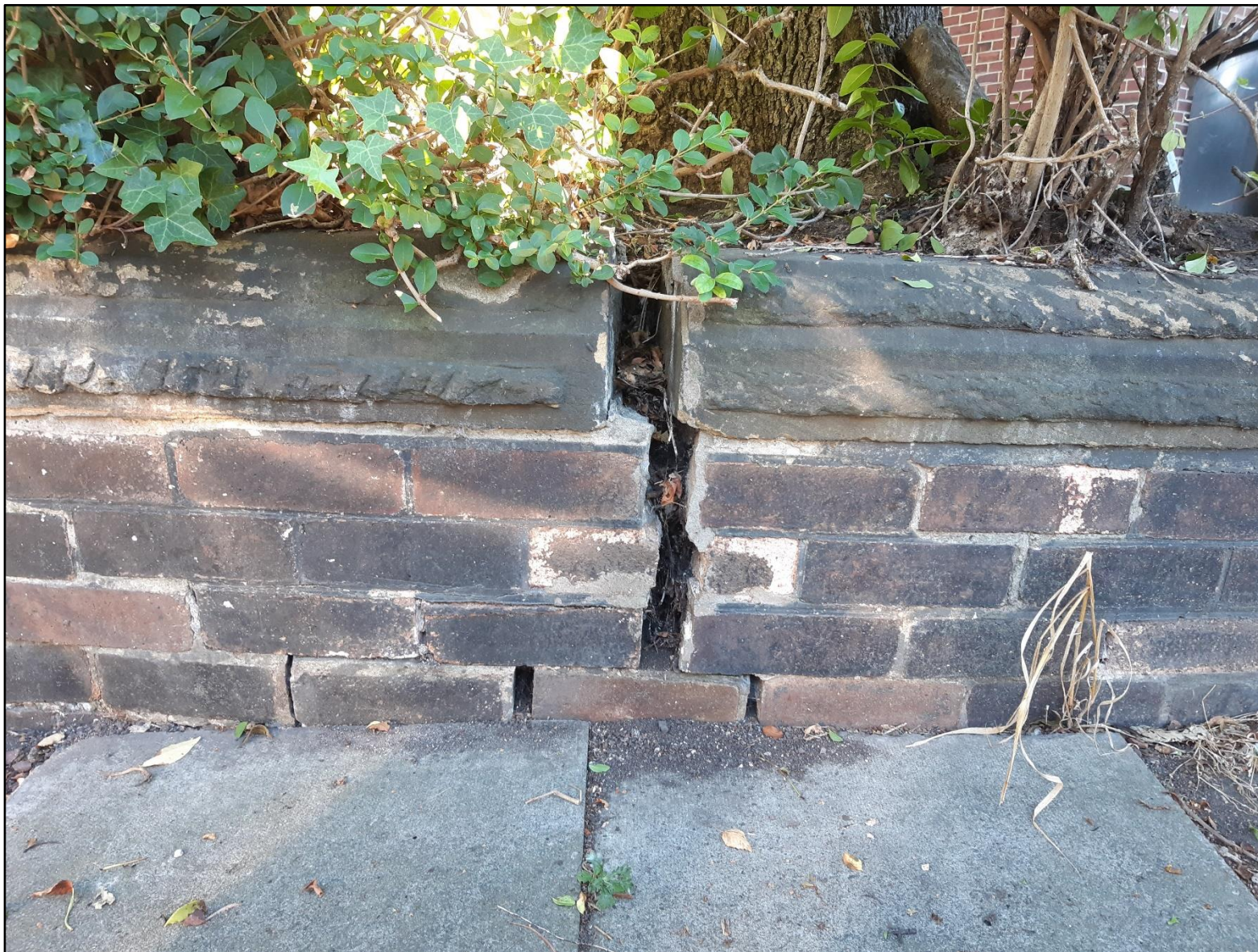
Photo 8 – Severe cracking in boundary wall attributed to tree
